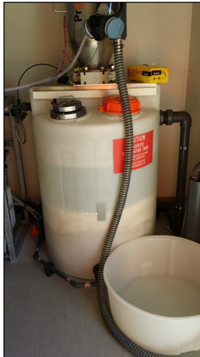
Figure 4-11: Fluoride System Saturator Tank
