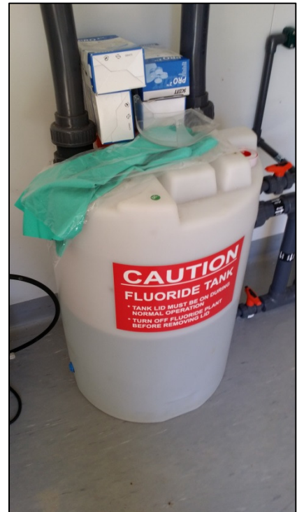
Figure 4-12: Fluoride System Dosing Solution Storage Tank
