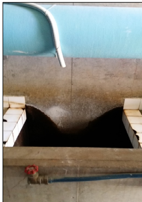
Figure 4-7: Post-Filtration Lime Dosing into Filtered Water Well for pH Correction
