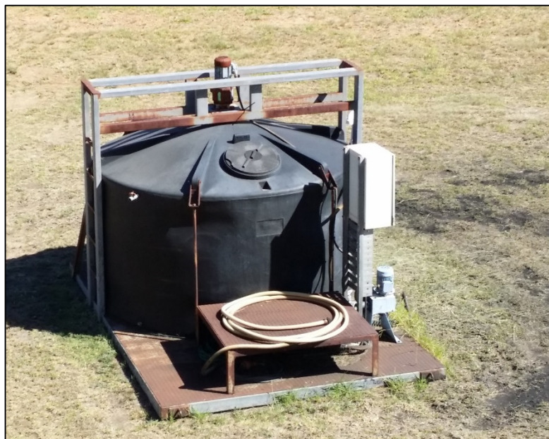
Figure 4-2: PAC Batching and Storage Tank at Coonabarabran WTP
