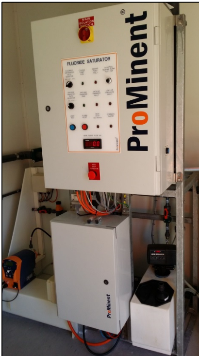
Figure 4-10: Fluoride System Control Panel and Water Softener
