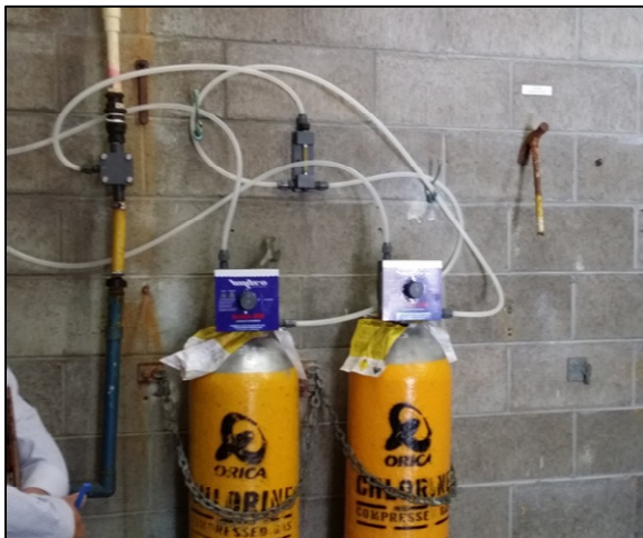
Figure 4-8: Chlorine Gas Dosing System Set Up
