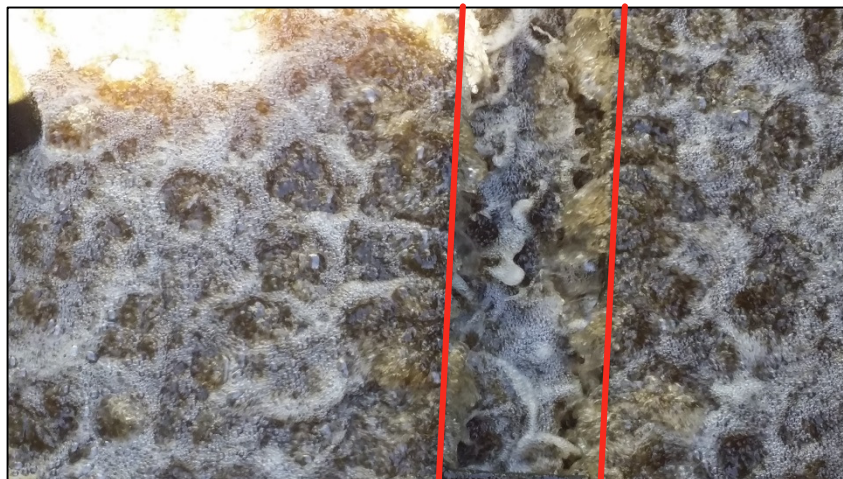
Figure 4-6: Air Scour Continuing During High Rate Water Wash Leading to a Loss of Filter Media
