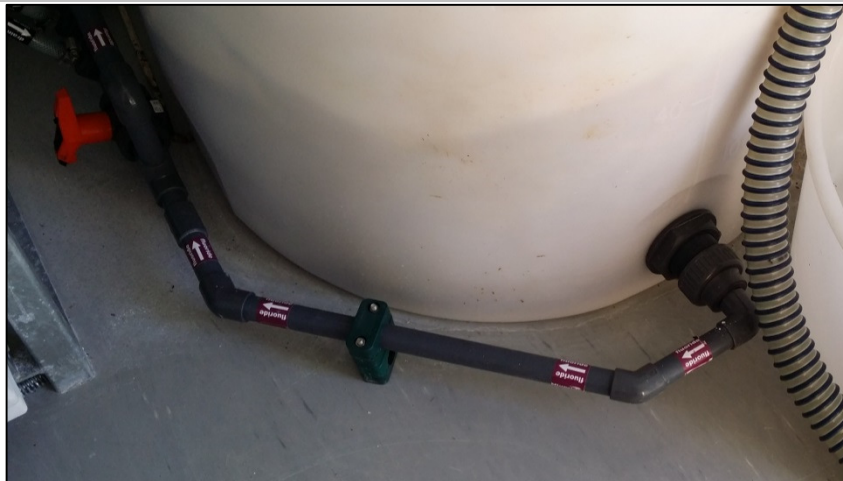
Figure 4-13: Outlet Pipework at Base of Fluoride Saturator Tank
